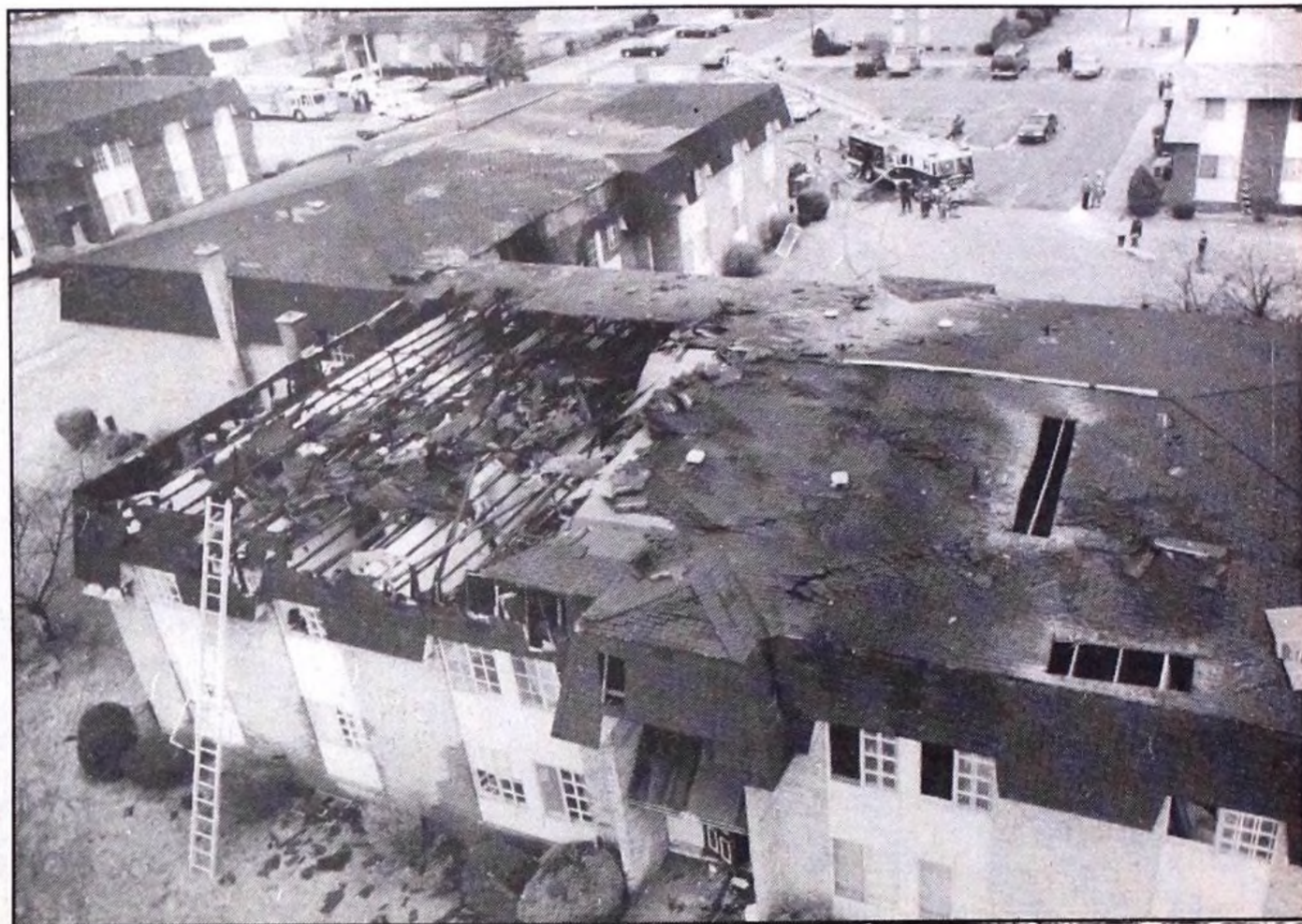
Firefighters battled the blaze at the Venoy Pines Apartment complex for more than two hours. ANP photo by George Riley
